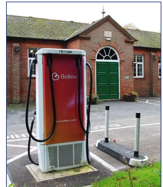
This charging point located at the Village Hall demonstrates how a communal location can be appropriate. Design should be considered to ensure that it does not detract from the existing historic character.
